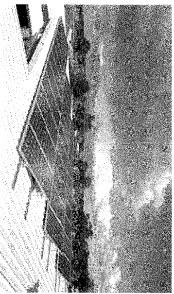
Solar Panels: Solar photovoltaic panels on the north side of the roof
