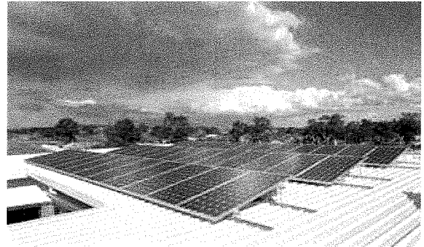
Solar Panels: Solar photovoltaic panels on the north side of the roof
