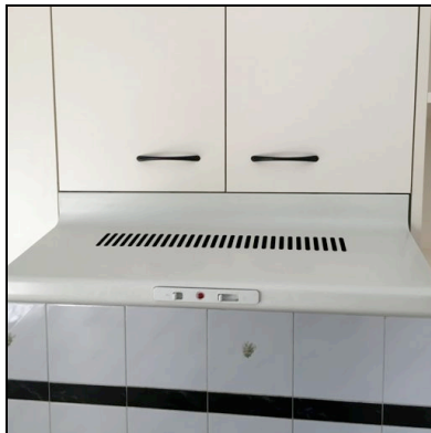
Photo No: 003 Rangehood
