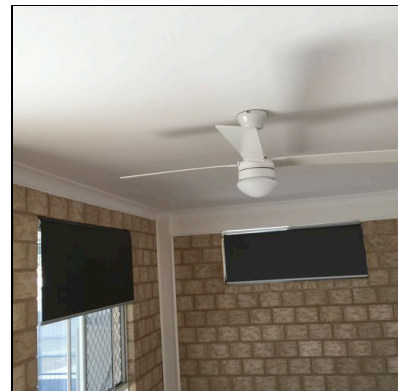
Photo No: 006 Typical Ceiling Fan
