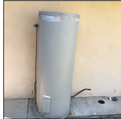
Photo No: 008 Hot Water System
