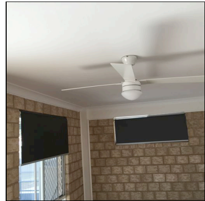
Photo No: 006 Typical Ceiling Fan
