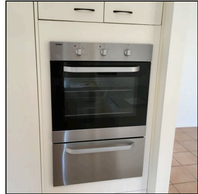
Photo No: 004 Oven
