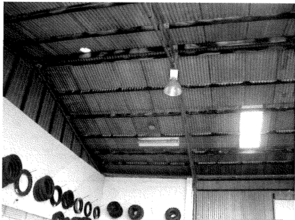
Lighting and skylight
