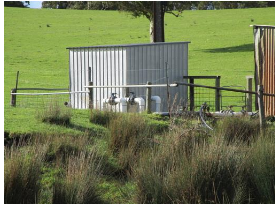
Irrigation pump shed
